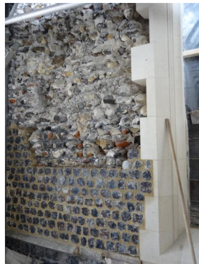
New stone work for the West Window and building up the knap-flint wall
