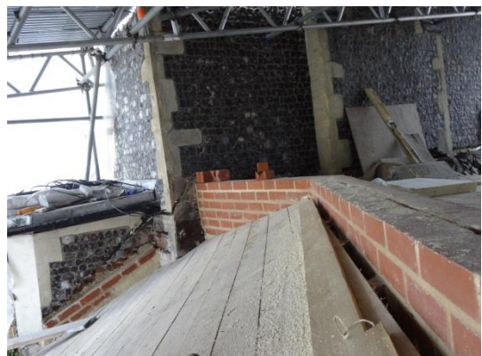
Sacristy area being rebuilt in preparation for new ceiling and roof and flint wall
